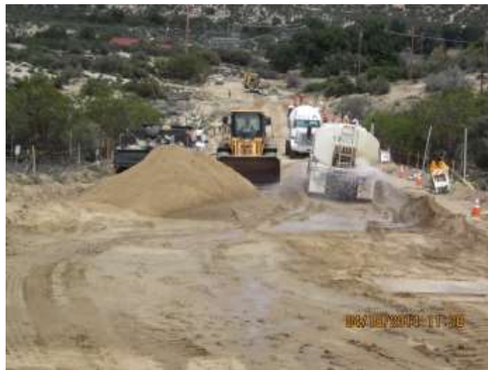
Photo 2: Water trucks being utilized during excavation and backfilling activities and along common used access roads to minimize fugitive dust emissions in accordance with the Dust Control Plan and MM-BIO-4a.
