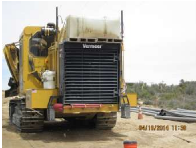
Photo 1: Drip pan containment bins beneath equipment staged along the right-of-way in accordance with MM-HAZ-1a.
