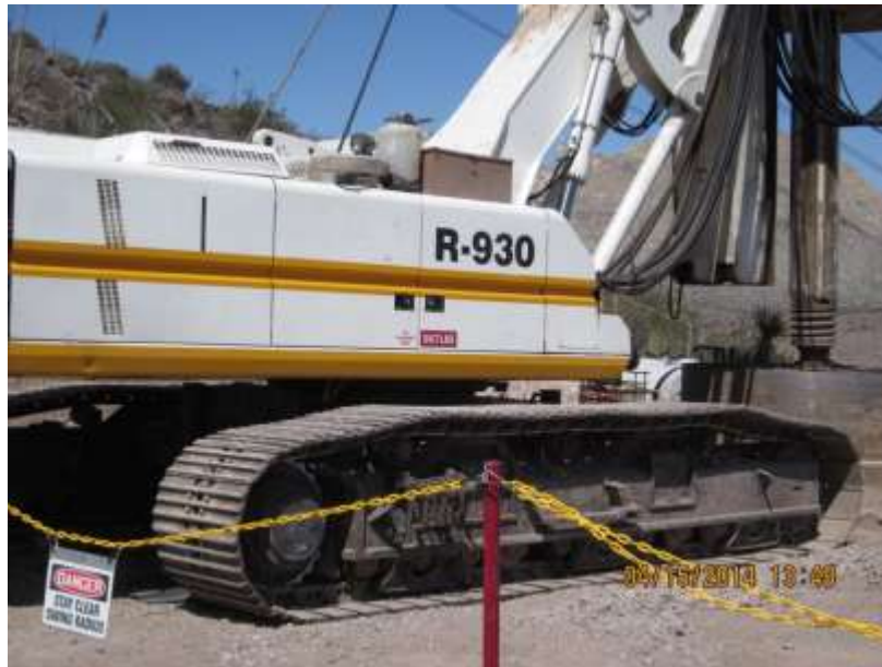
Photo 5: Routine patrols were completed by the fire inspection team throughout the construction activities and fire tools were observed at all construction sites as required by MM-FF-1.
